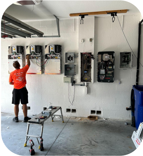
Battery storage for a 4.62 kW rooftop solar array with back-up battery.
