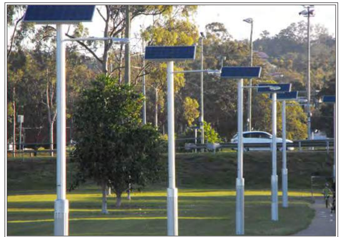
Lighting and electrical distribution infrastructure can minimize El Paso's citizens to exposure to electrocution and other hazards by hiding wires and by incorporating on-site energy generation. Off-grid infrastructure is also less-polluting. Image courtesy of Multipole Global.
