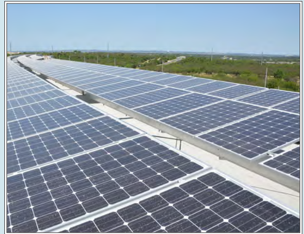
Project done by Texas Solar Power Company, Austin, TX
